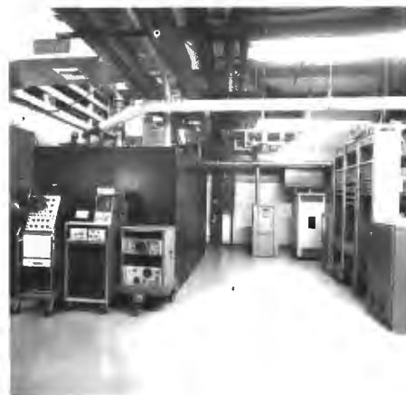
The entire TV-39 transmitting plant is maintained in impeccable condition, as this view of the rear cabinet area shows.
