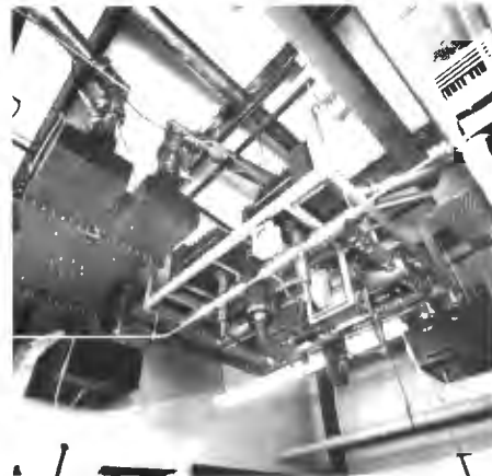
A portion of the ceiling mounted equipment, including waveguide transmitter combining system and one of the two filterplexers used in the system.
