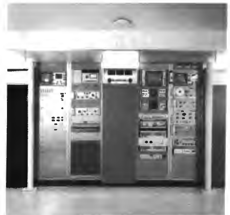
Control and monitoring racks. Center unit is parallel control cabinet for total system aural and visual output, and for automatic exciter switching. Other racks mount audio and video input monitoring and remote control equipment. System layout was designed by Transmitter Supervisor Bill Stevens.
